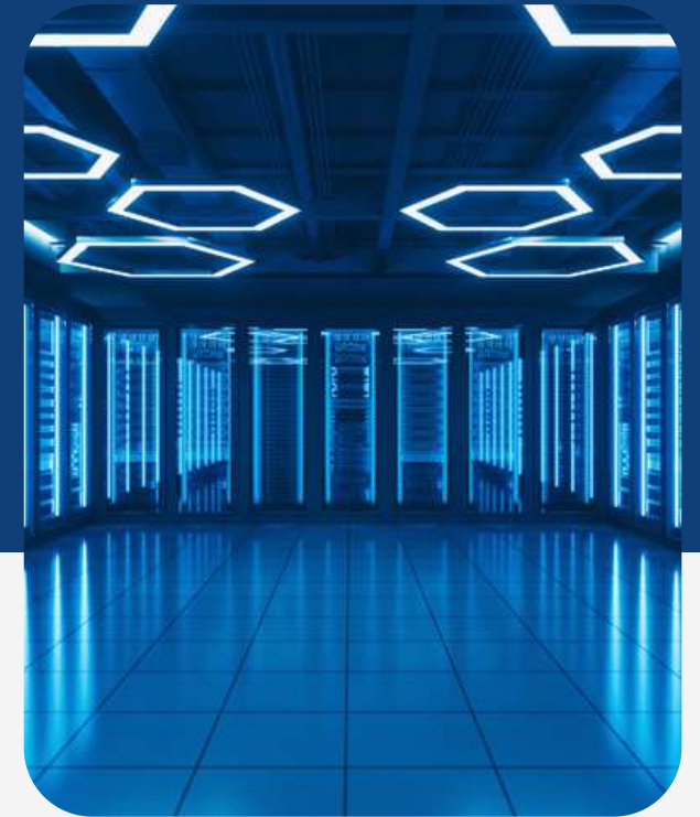
5. Data Centre Equipment
